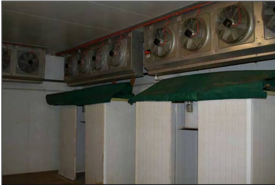
Plate 3. Tunnel cooling showing reinforced blind which is run over and down the end of the air channel
