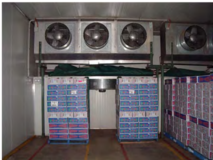
Plate 1. Cool room with forced air fans for rapid and uniform cooling.
