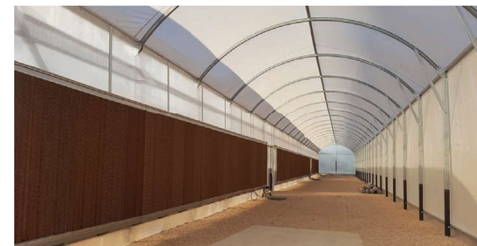
Cooling pads in the new facility.
