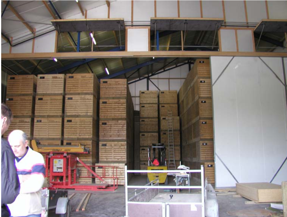
Figure 2: Store room for onions and potatoes designed with a drying wall system.
