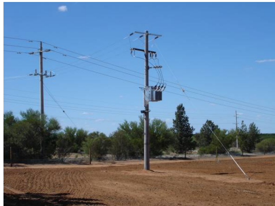
Figure 3 Power pole and transformer
