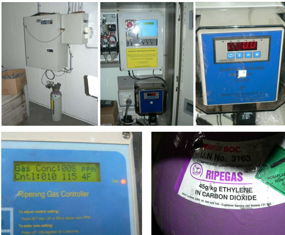
Figure 2. Real-time ethylene monitoring and delivery equipment installed in two ripening facilities. The system uses RipeGas ® (BOC Limited) as a dilute form of ethylene ( \cong 6-8%), and monitors and controls CO 2 to prevent accumulation to quantities that may be dangerous to personnel and cause damage to fruit.
