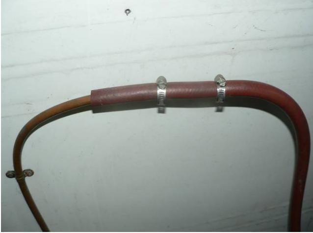
Figure 5. Non-optimal plumbing for pulse delivery ethylene system.
