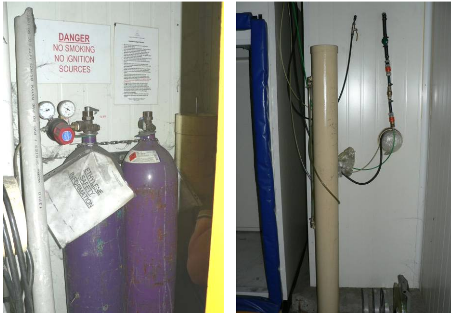
Figure 3. Pulse ethylene delivery equipment installed in two ripening facilities. The system passes pure ethylene through a water tower to mix and humidify the gas. Ethylene pulses are delivered at intervals predetermined by the system installation staff. This system does not monitor the actual ethylene concentrations in the ripening room.
